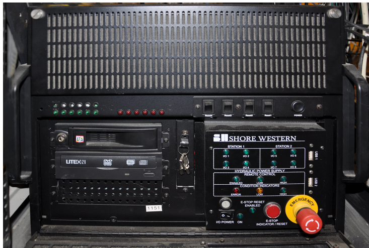
Figure 2.26: Shore Western SC6000 Controller
